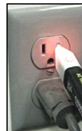
AC Voltage in wall receptacles
