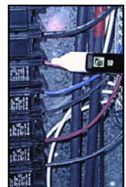
AC Voltage in junction boxes
