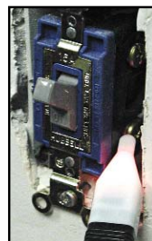
AC Voltage in switches
